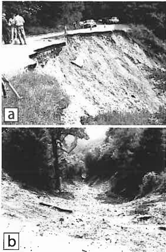
Figure 2. (a) Initiation site of road-fill failure (milepost 348.8) and (b) downslope impacts from debris flow. Arc-shaped pavement crack at initiation site was evident months prior to failure in September 2004. Photos courtesy of the Federal Highway Administration.
